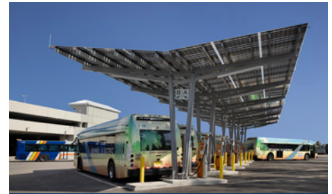
Ravenswood Bus Charging Infrastructure
