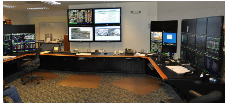
Existing Main Control Room
