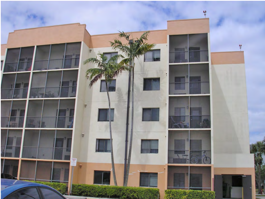
P26 8210 South Section Unrepaired Walls
