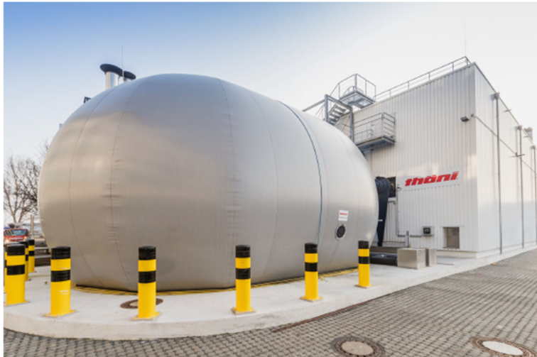
Biogas Storage at Anaerobic Digestion Plant, Frankfurt, Germany
