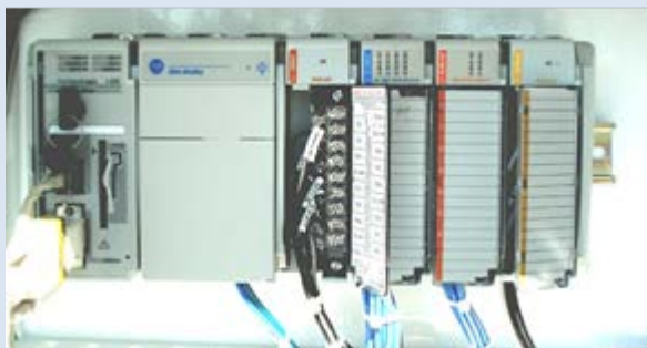
Allen Bradley Compact Logix PLC
