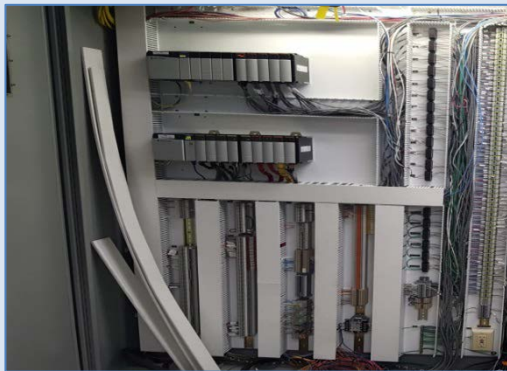
Control Logix PLC AFTER
